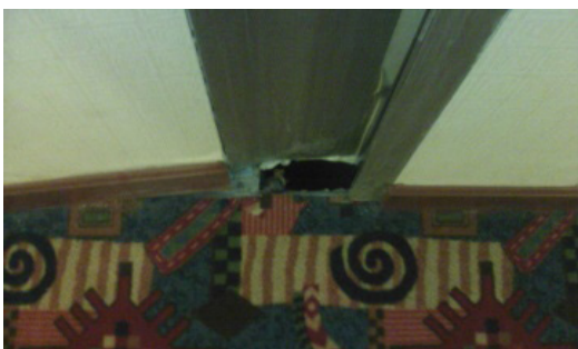
Figure 4: Damage caused by earthquake
