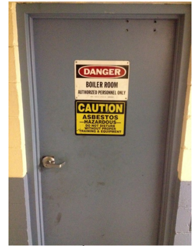
Figure 3: Asbestos Caution Sign Posted at Hilton Anchorage
