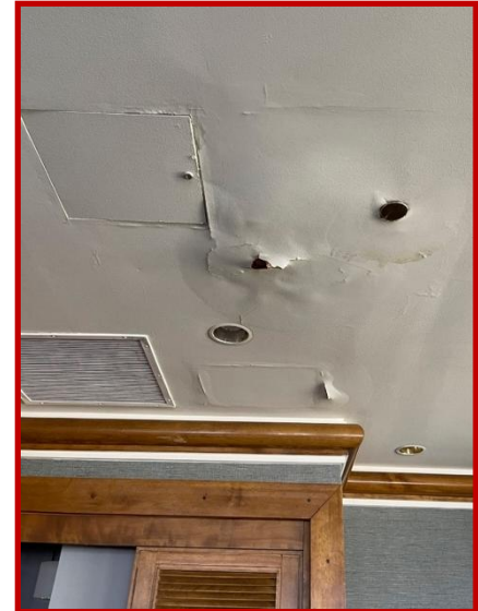
Ceiling damage near Top of the World Restaurant 8/5/2021
